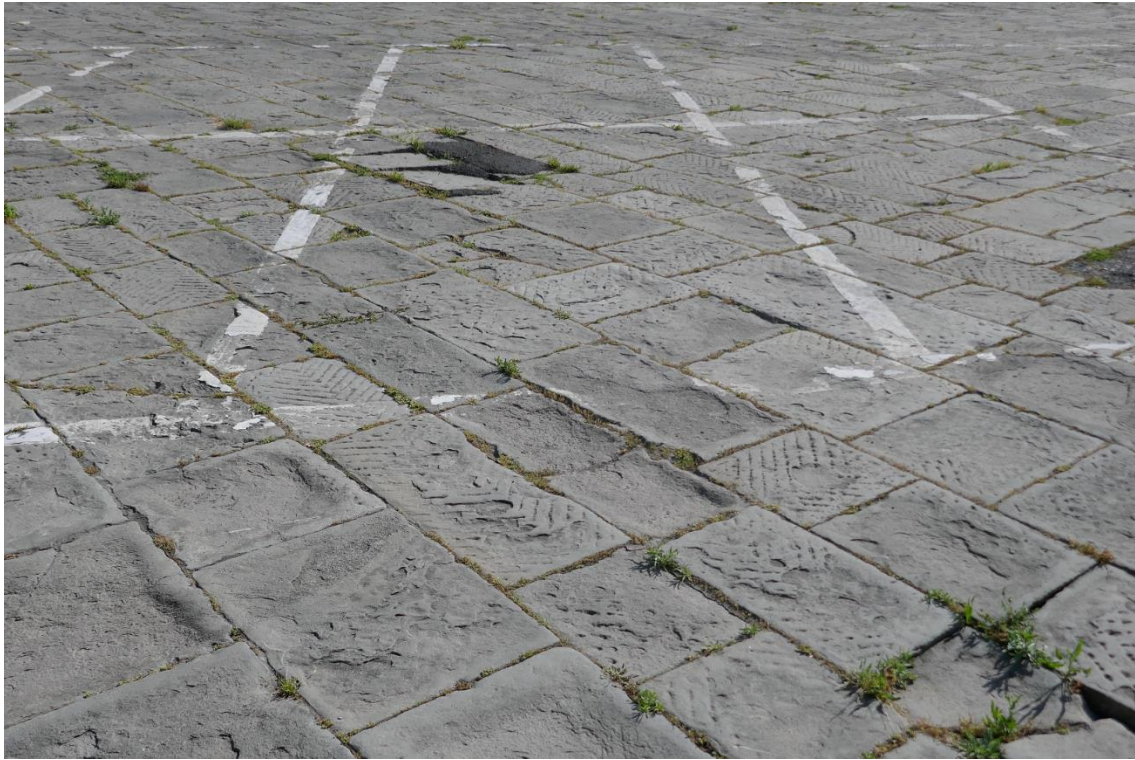
Fig 14 Traditional paving of the Nuova Piazza del Carmine awaiting repair
