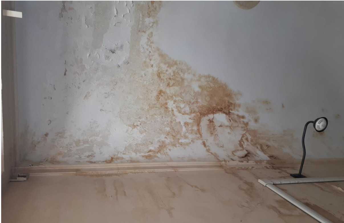
Fig 22 One of the top floor front rooms in the San Firenze complex, showing signs of past water ingress behind the parapet of the central block, prior to re-covering the roof
