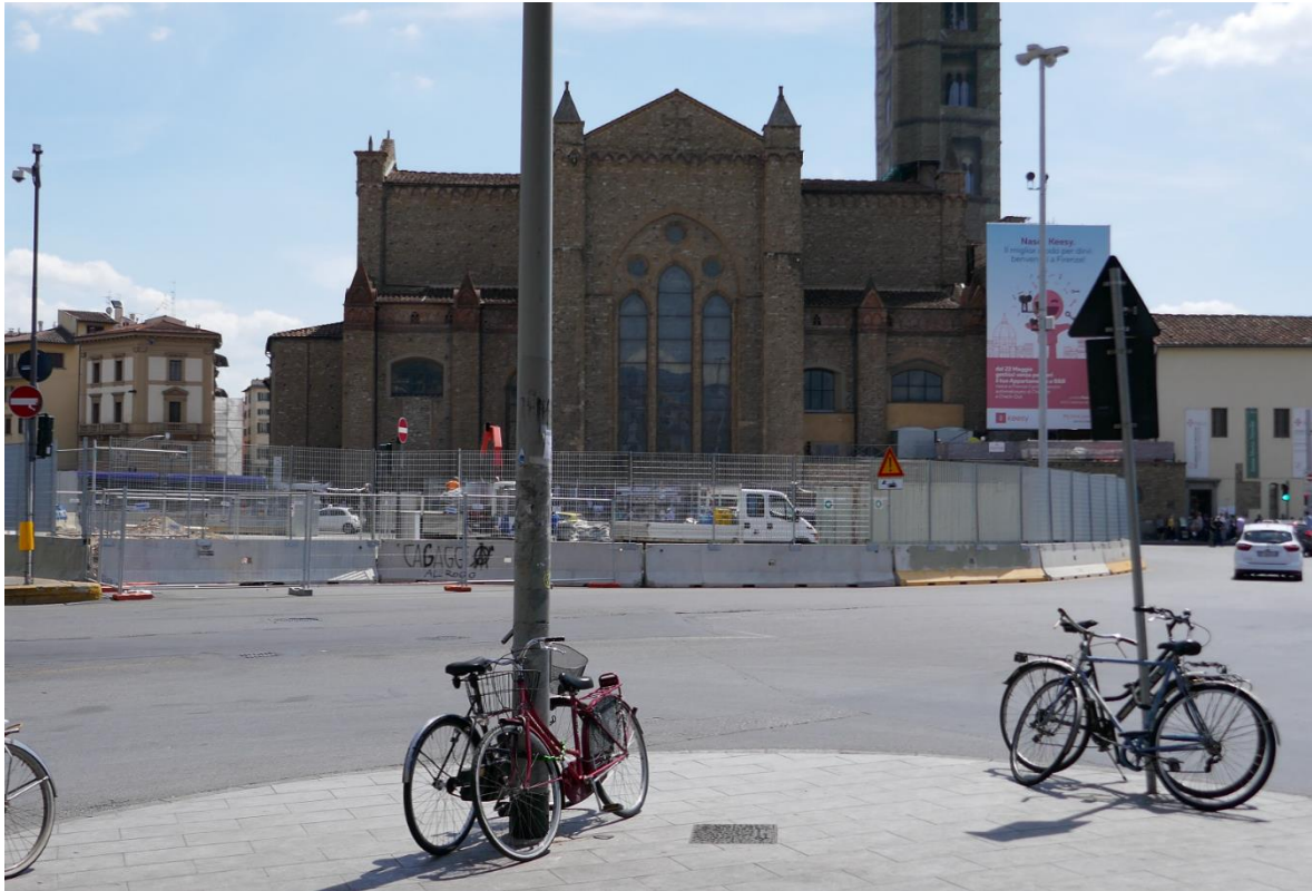
Fig 12 Tramway construction work with the gable of Santa Maria Novella in the background
